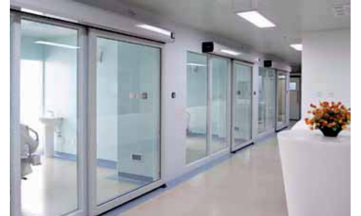
Clear View glass hermetic doors. Hospital ICU room.
